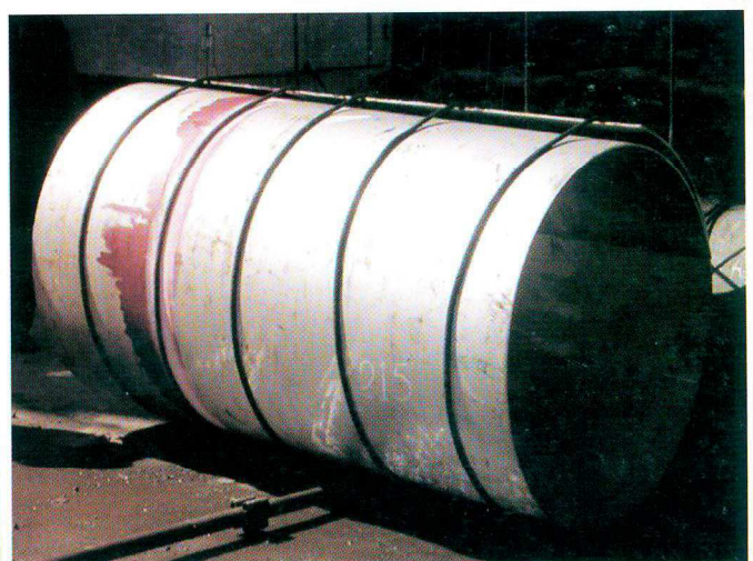
Picture 4. Rolled lining ready for insertion into the neck of a vessel.
